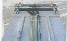
Top hydraulic pipeline
