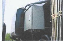
PLC Modular control box
