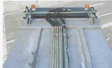
Top hydraulic pipeline
