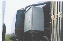
PLC Modular control box
